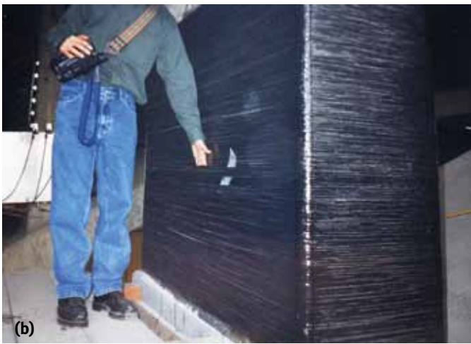
Fig. 4: Signs of poor installation techniques: (a) bubbles and sagging fibers; and (b) large voids
