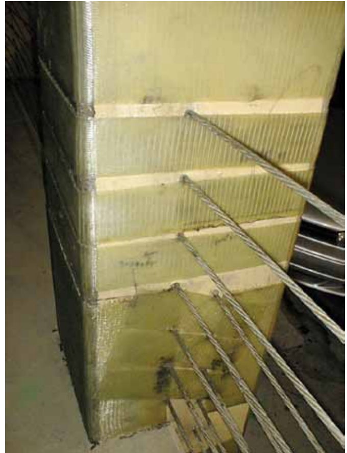
Fig. 3: This GFRP system was poorly installed around the barrier cables; it was subsequently removed and replaced
