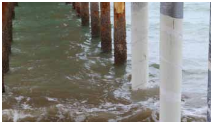
Fig. 5: Retrofit of underwater piles, from top to bottom: construction of a seamless jacket with super laminates; filling the annular space; and completed pile jacket
