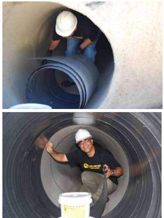
Fig. 2: Super laminate being taken into the pipe and installed; one size fits all pipe diameters
